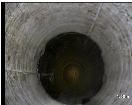
Observation [5]: patch liner end
